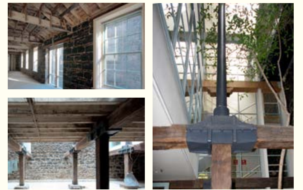
The original open internal structure of -573- is revealed when John Wardle Architects were contracted to revive its heritage for Arnold Thomas & Becker Lawyers. JOHN HORTON & JOHN WARDLE ARCHITECTS
